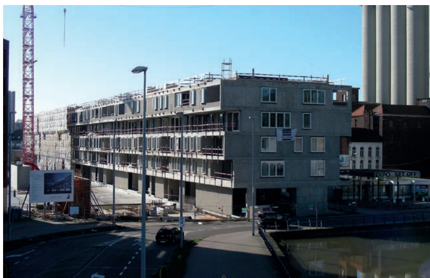
"De Balk van Beel" apartment building in Leuven, Belgium where a smart energy management system is being installed
