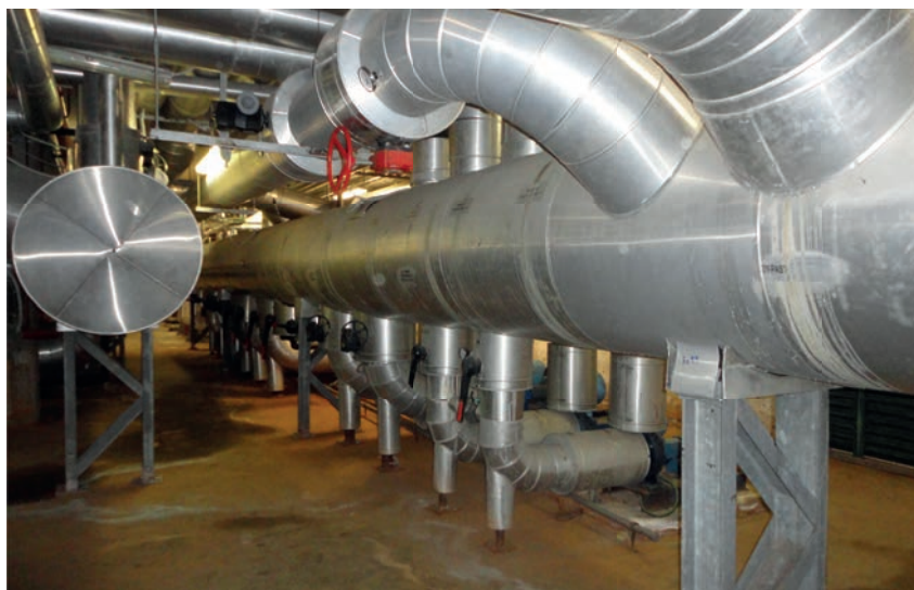
Chilled water distribution pipes at Fiumicino airport
